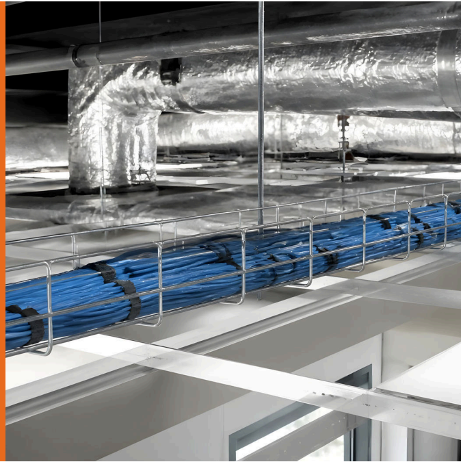
Commercial TI: structured cabling above an accessible ceiling
