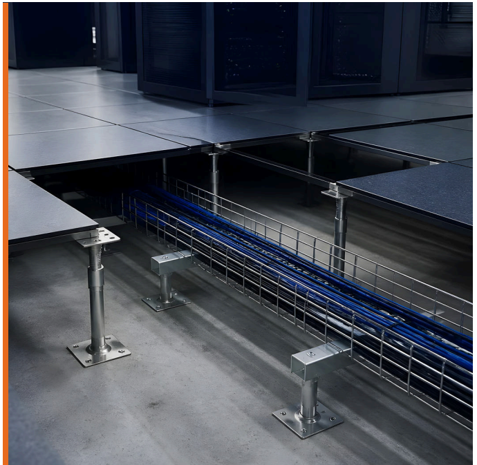
Raised floor: tray on floor stands between the pedestals
