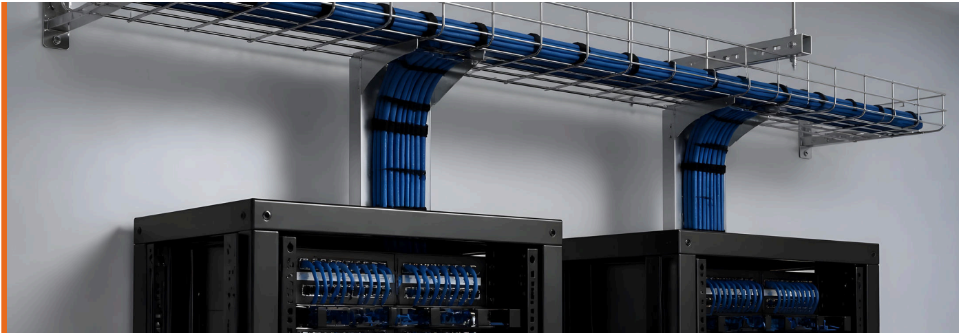
APPLICATION Telecom room: wall bracket and trapeze-supported tray with waterfall drops into each rack
