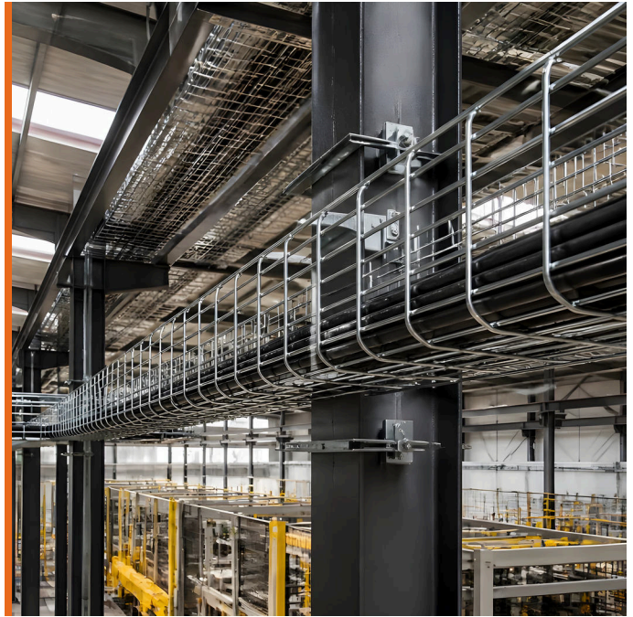
Industrial: hot-dip galvanized tray on columns and beam clamps
