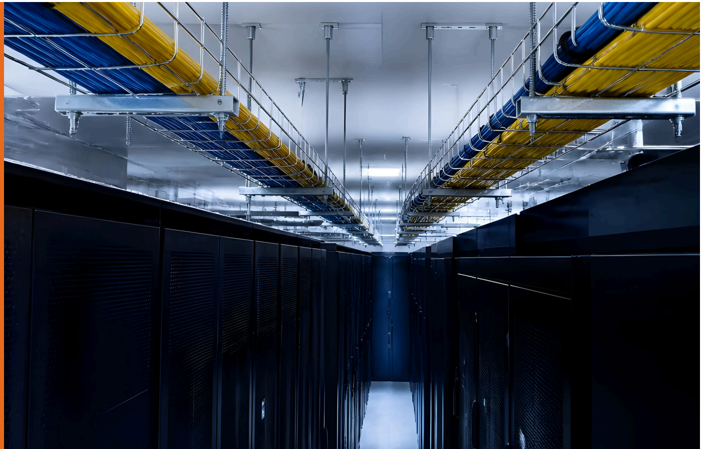
APPLICATION Data center hot aisle: parallel tray runs on strut trapeze hangers above the cabinets
