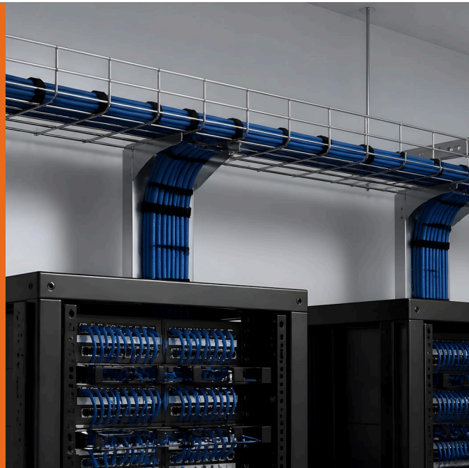
Telecom room: wall bracket and trapeze support, waterfall drops into the racks
