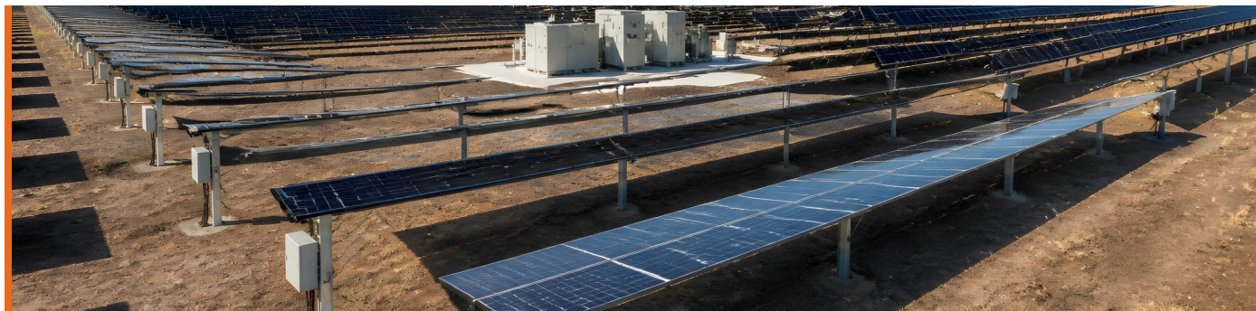
APPLICATION 1500 V tracker rows: combiners on the piles, string harnesses on messenger wire, central inverter skid
