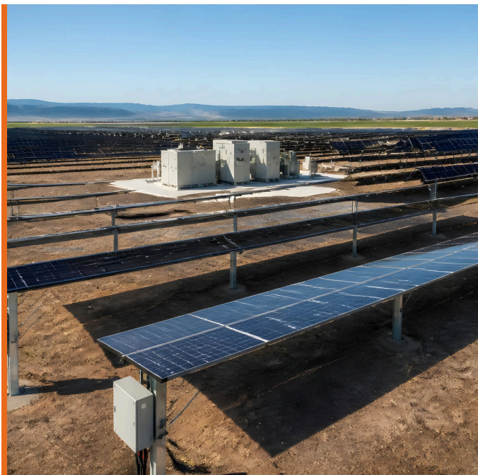
Utility 1500 V: pile-mounted combiners and messenger-wire string harnesses
