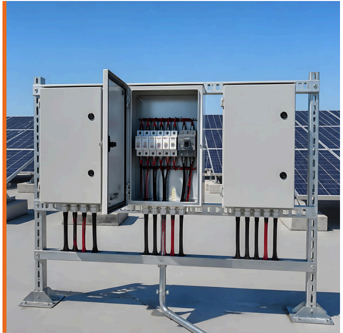
Commercial roof: steel combiners on a strut frame, bottom cable entry
