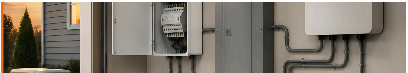
APPLICATION Automatic transfer switch between the main panel, hybrid inverter, batteries and a standby generator
