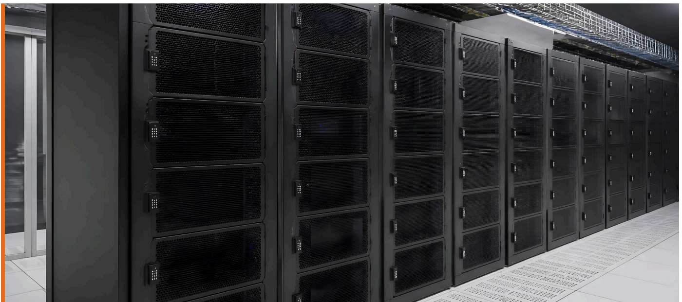
APPLICATION Bayed cabinet rows in a colocation data hall
