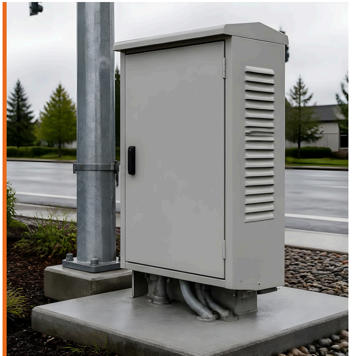
Outdoor: pad-mounted cabinet with sealed conduit entry
