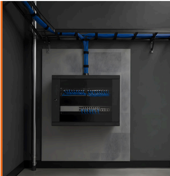
IDF: wall-mount cabinet on a plywood backboard
