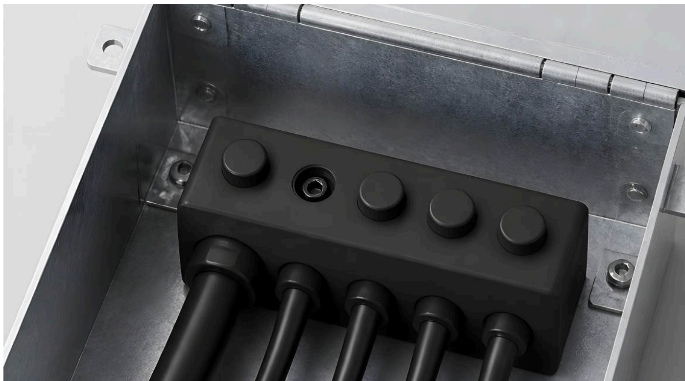
Application: insulated multi-tap connectors in a gutter and pull box.
