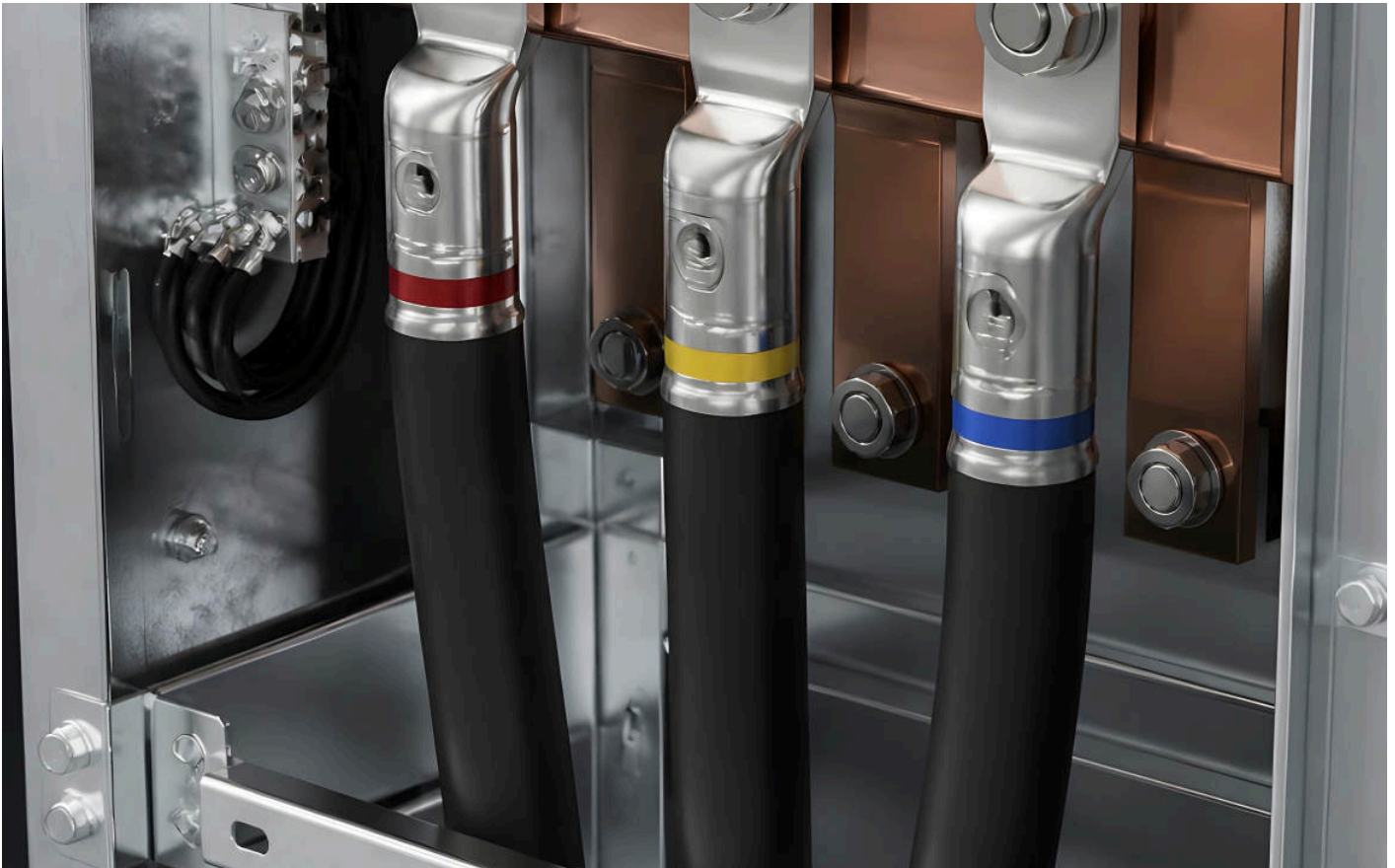
Application: compression lugs landed on panelboard and switchgear bus.
