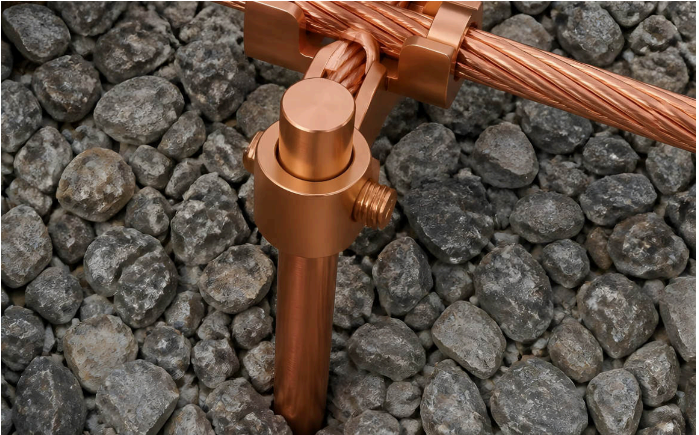
Application: buried grounding grid joined with irreversible compression connectors.
