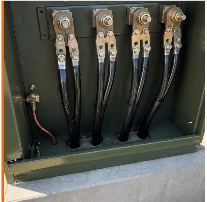
Pad-mount secondary: multi-hole spade terminals on the stud bushings, cable lugs bolted on 1-3/4 in. NEMA spacing
