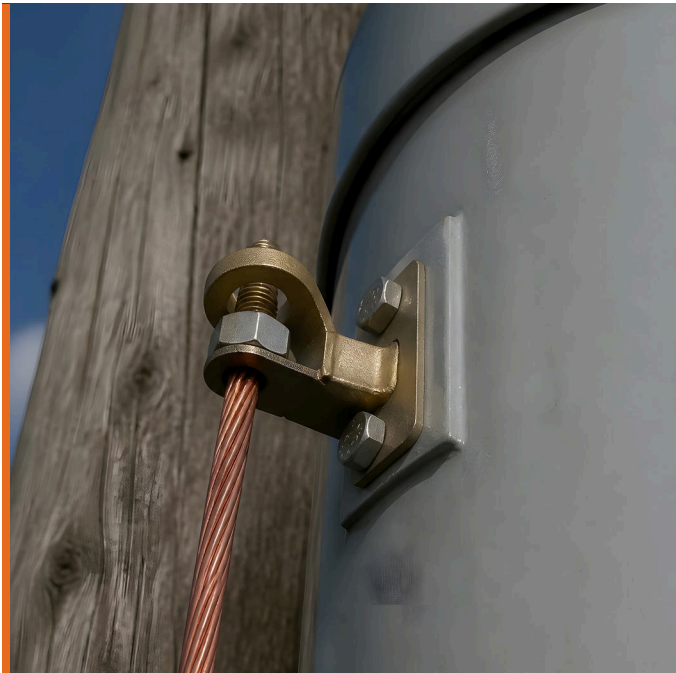
Tank ground: 90° bronze clamp on the tank ground pad, bare copper lead to the pole down-lead and system neutral
