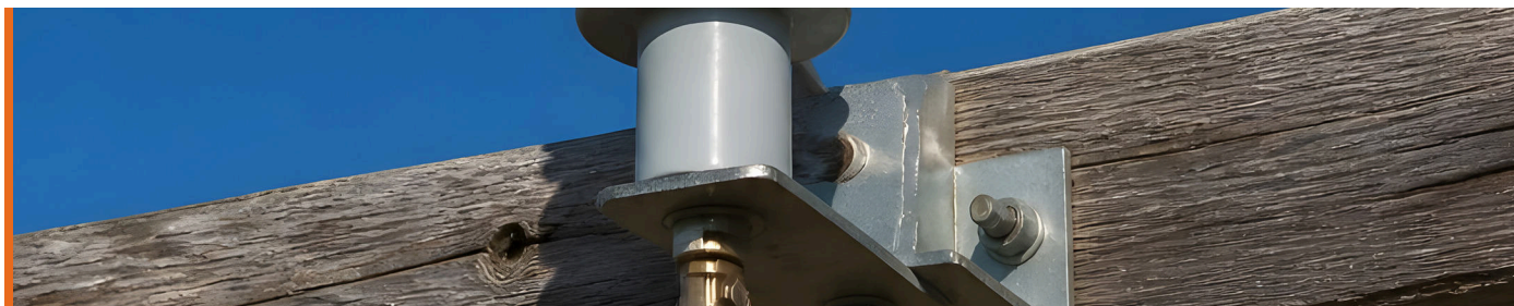
APPLICATION Arrester on the crossarm: bronze ground terminal on the bottom stud, bare copper lead to the pole ground
