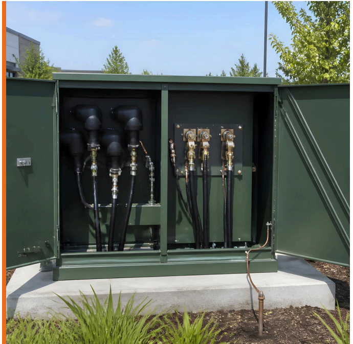
Underground residential and commercial: pad-mounted transformers with spade terminals and tank grounds
