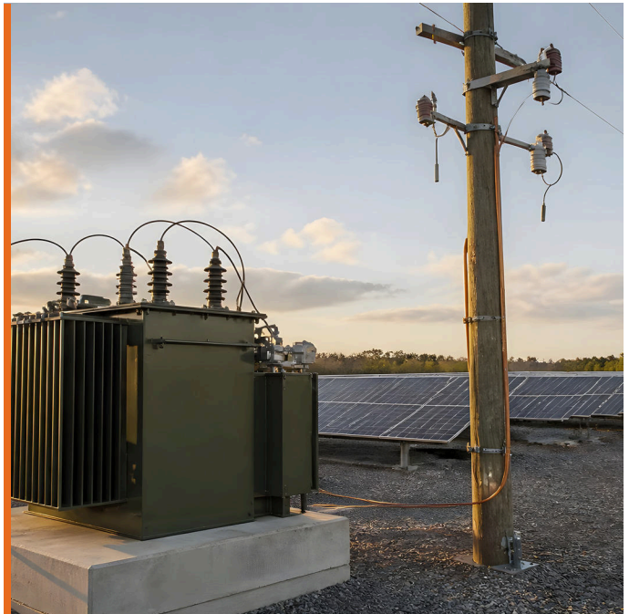
Renewables: solar and storage interconnections with riser-pole cutouts, arresters and grounding
